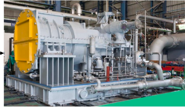
(2) Steam Turbine Generator
