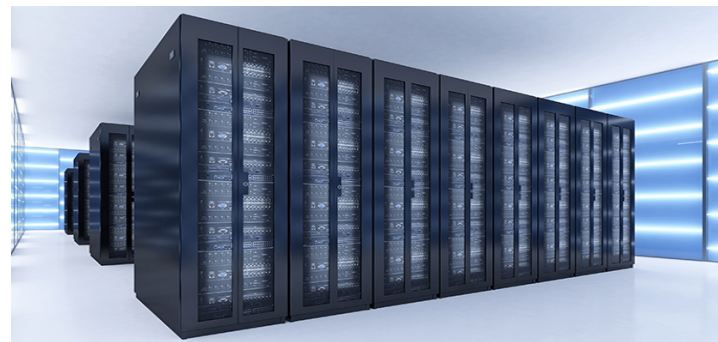
Data Center AI Server Racks
