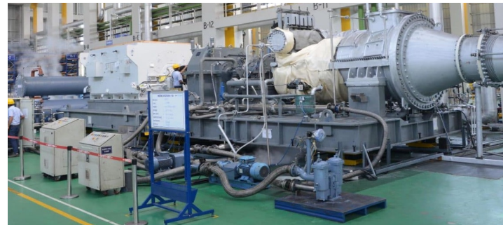
Turbine Power Plant
